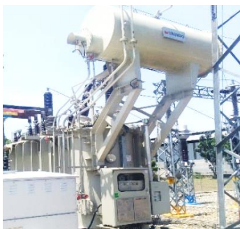
Gambar 6. Trafo type UNINDO 906007289
